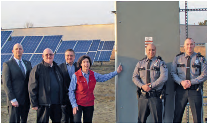
East Windsor officials “turn the switch” on newly constructed solar system array to power the Township Police/Court facility. Pictured (from left to right) are: Chief of Police James Geary; Council Member Alan Rosenberg; Council Member John Zoller; Mayor Janice S. Mironov; Police Officer Danny Fernandez, and Police Officer Gregory Hager.
